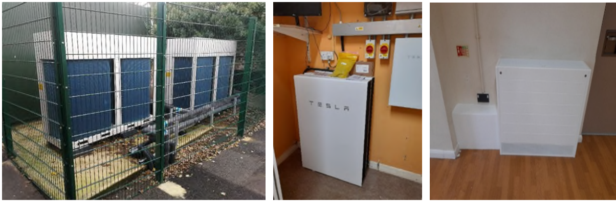
Ninfield school: air source heat pumps; battery storage; new radiators.
